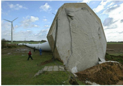
Figure 6: Example of a toppled wind turbine (Nova Scotia Power's Nuttby Mountain) https://ontario-wind-resistance.org/2011/02/03/nearly-all-22-turbine-foundations-cracked/ .
